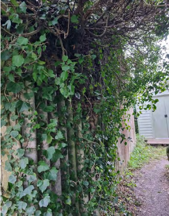
Photograph 9: Close up of the exterior of one of the existing barns, overgrown with foliage. Potential ACMs are present within the barn's building fabric.
