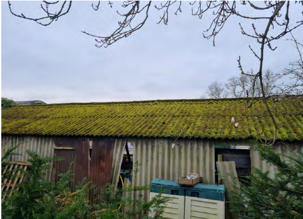
Photograph 3: Exterior / rear elevation of one of the barns, shown to be in a partially dilapidated state. Potential ACMs are present within the barn's building fabric.
