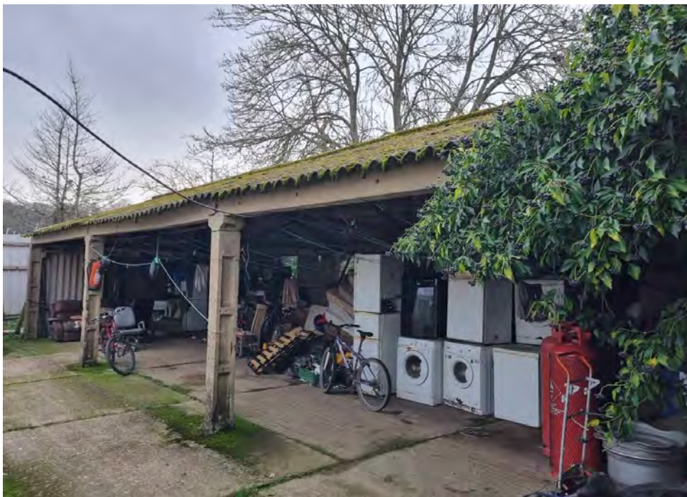
Photograph 2: Open-sided storage barn located on-Site, including some domestic white goods and objects, as well as two gas tanks, located in the east of the Site. Potential ACMs are present within the barn's building fabric.
