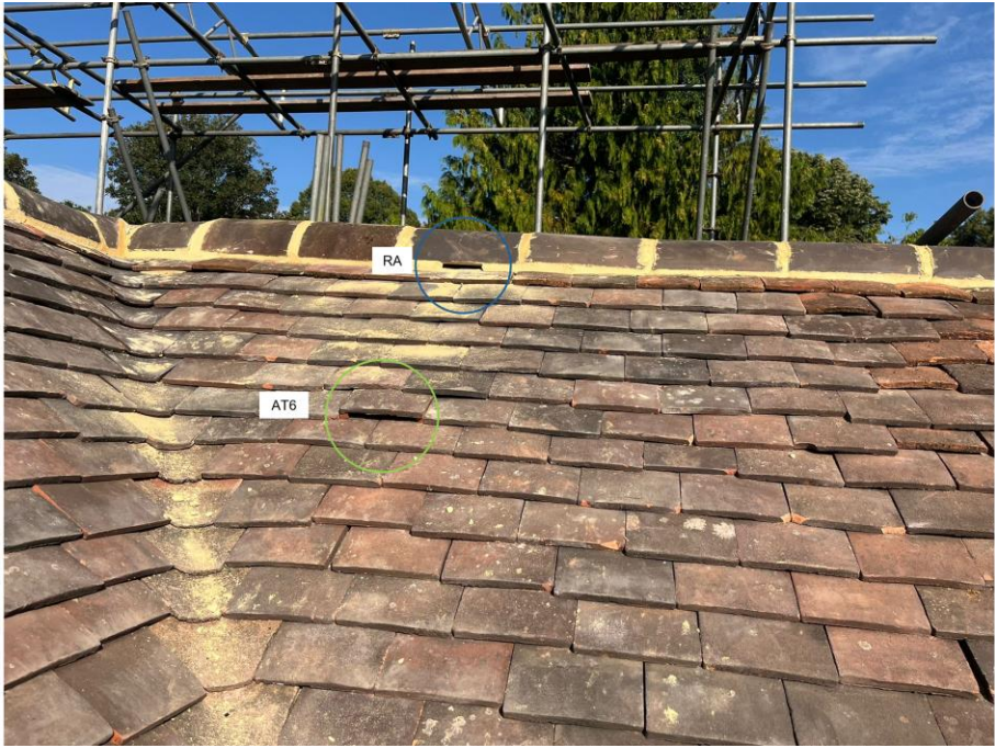
Figure 4 - Bat Access Provisions on Rear Flank of Front Roof
