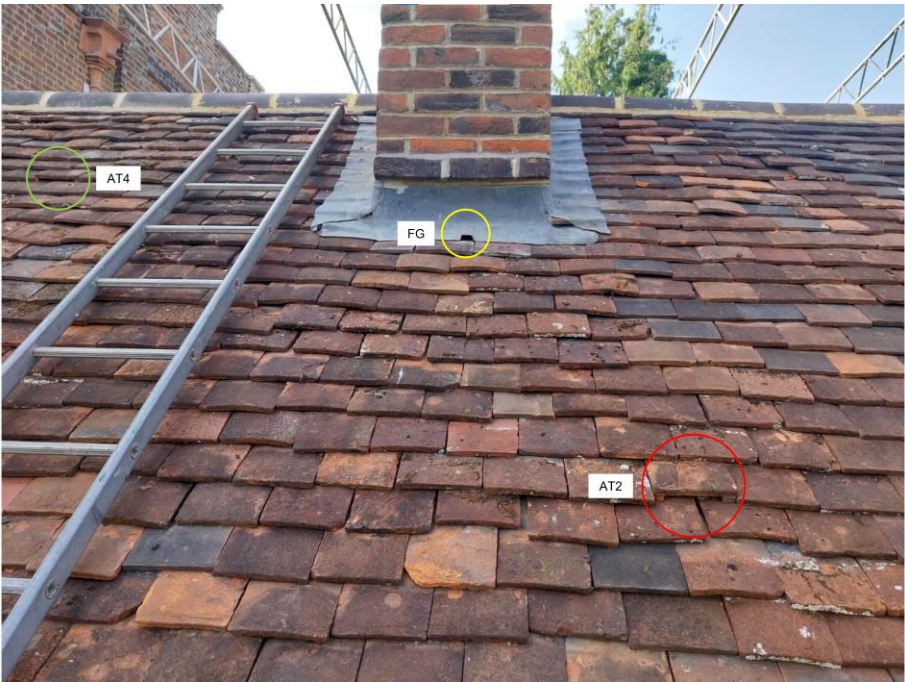
Figure 6 - View of Chimney Flashing Gap
