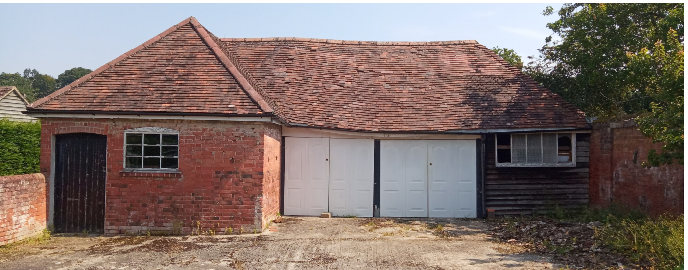
C) Front elevation of store building showing existing white powder-coated aluminium garage doors with raised and fielded panels, which are not historically consistent in terms of material or panel profiles.
