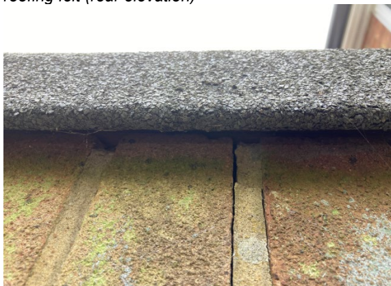
Photograph 11. Gap between flat roof and garage wall
