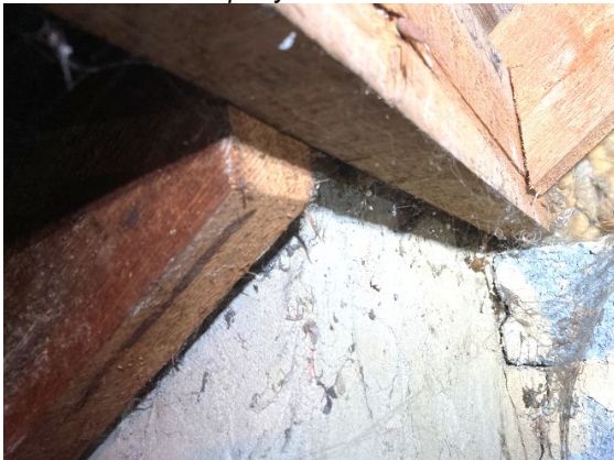
Photograph 19. Tightly fitted cemented chimney with cobwebs (western elevation)
