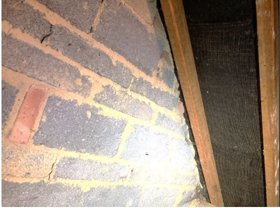
Photograph 17. Cobwebbed gap along the edge of the western blockwork party wall.
