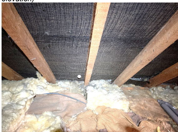
Photograph 16. Fibreglass filled eaves and torn bitumen felt
