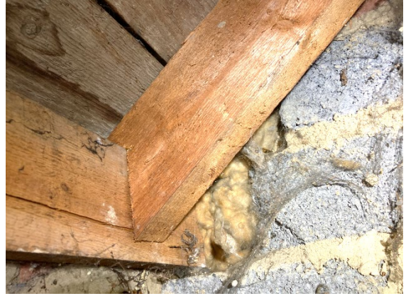
Photograph 18. Gaps in blockwork, filled with fibreglass insulation on the party wall.
