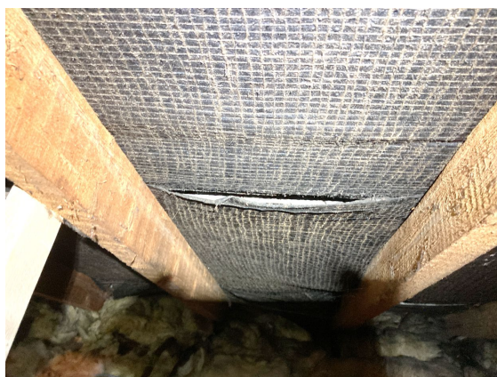
Photograph 15. Loosely fitted bitumen felt (eastern elevation)
