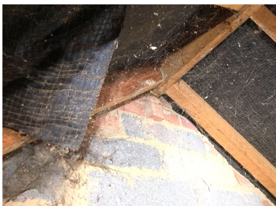
Photograph 14. Loosely fitted bitumen felt (western elevation)
