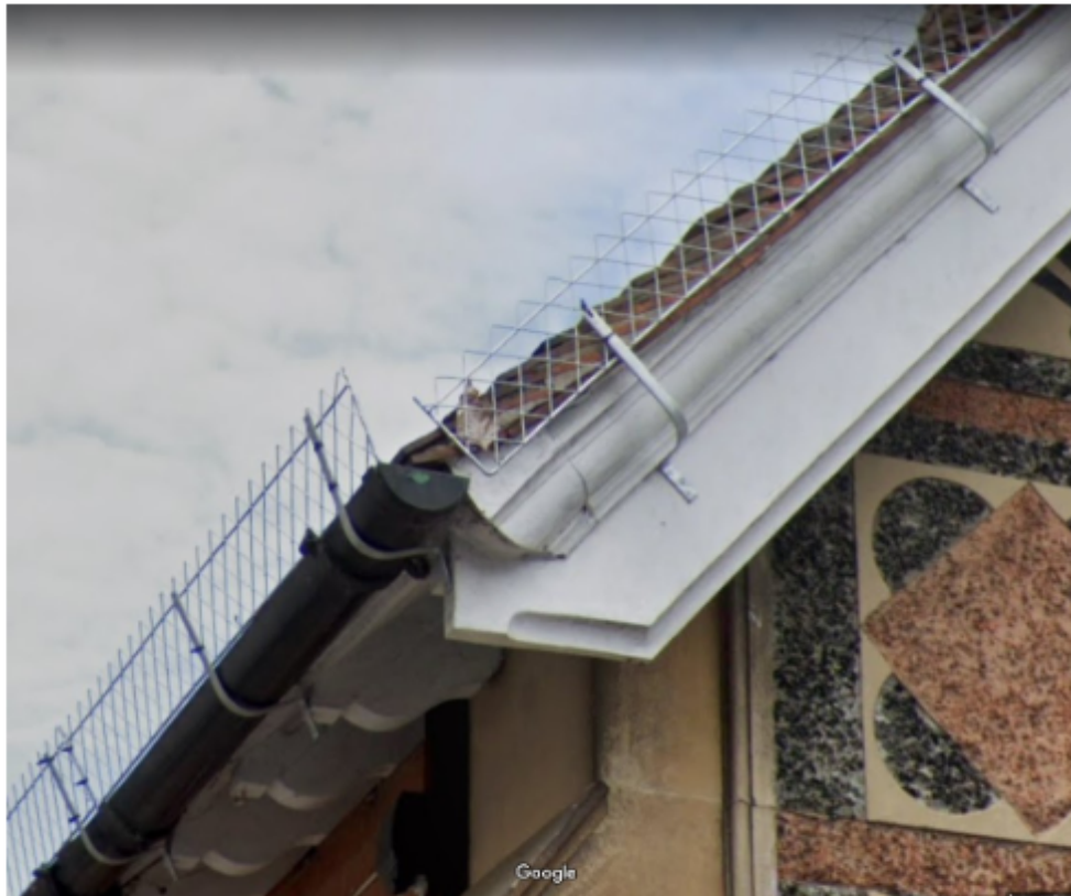
Metal Mesh Snow Guard system attached to building.
