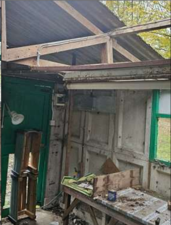
TN 14: Wooden outbuilding interior with missing roofing.
