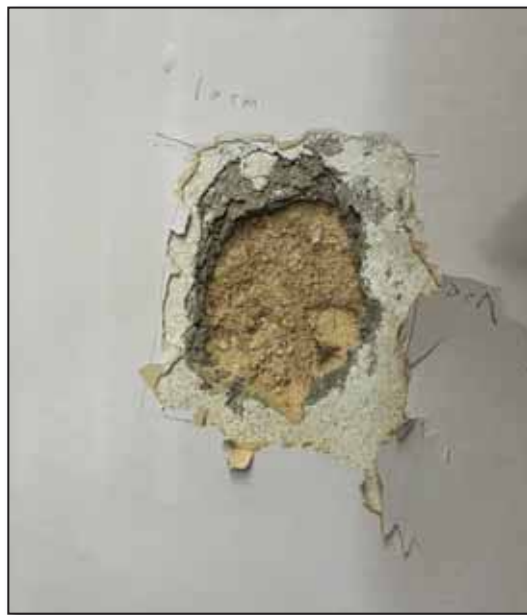
Image 17: Exposed area of fabric
