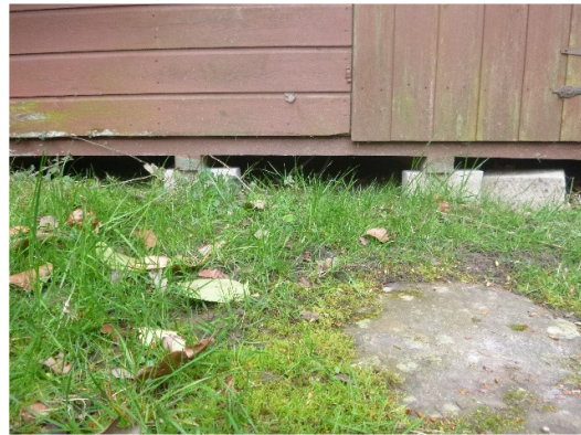
Photograph 16. Gaps under the shed by the rear of the house.
