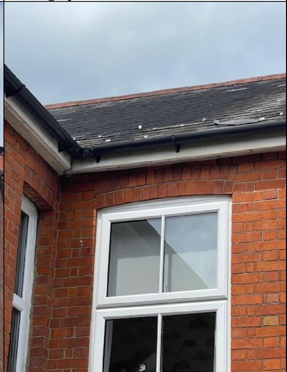
Photograph 4: Gaps around wooden soffits.
