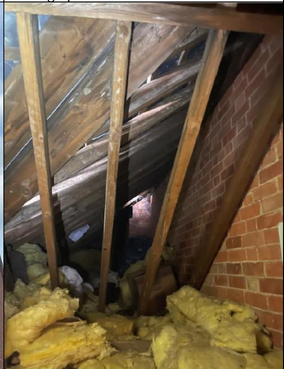
Photograph 8: Loft space, gaps in tiles.
