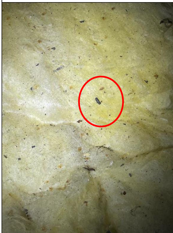
Photograph 11: Bat droppings found within the loft space.
