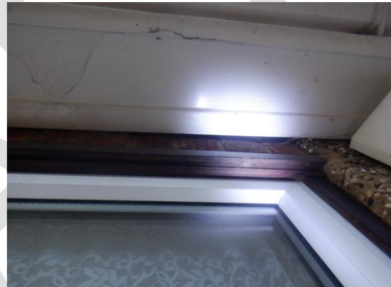
Photograph 9. Gap between uPVC soffit & brickwork (front elevation).
