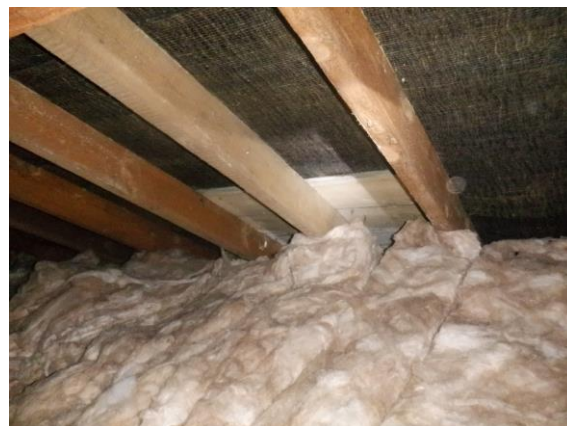
Photograph 12. Bitumen felt tight to the chimney timbers.
