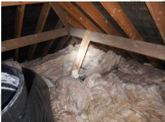
Photograph 13. Eaves blocked by fibreglass insulation.
