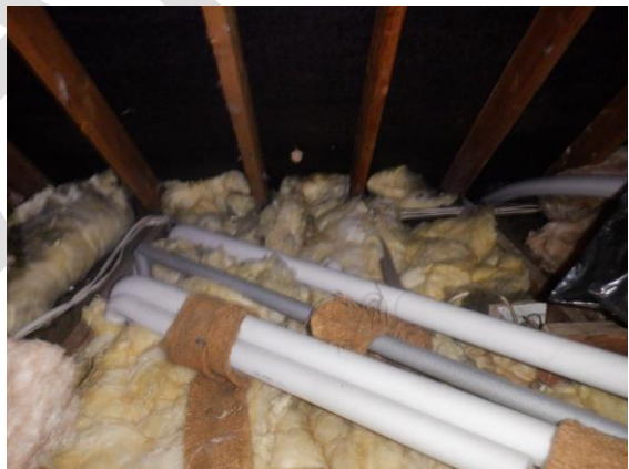
Photograph 14. Small in-active wasp nest within southwest corner of the void.
