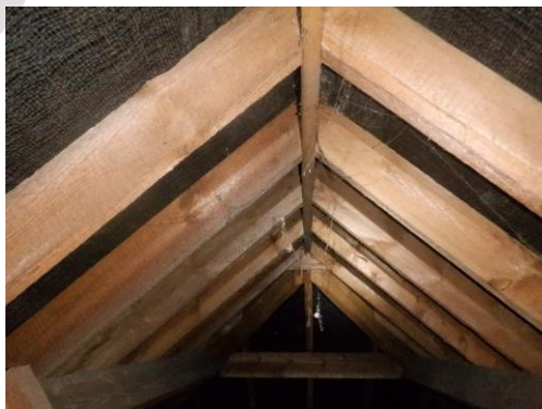
Photograph 10. Ridge cobwebbed throughout the void.
