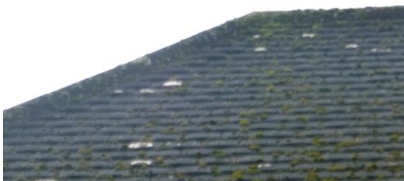
Photograph 3. Lifted clay roof tiles along the hips (rear elevation).
