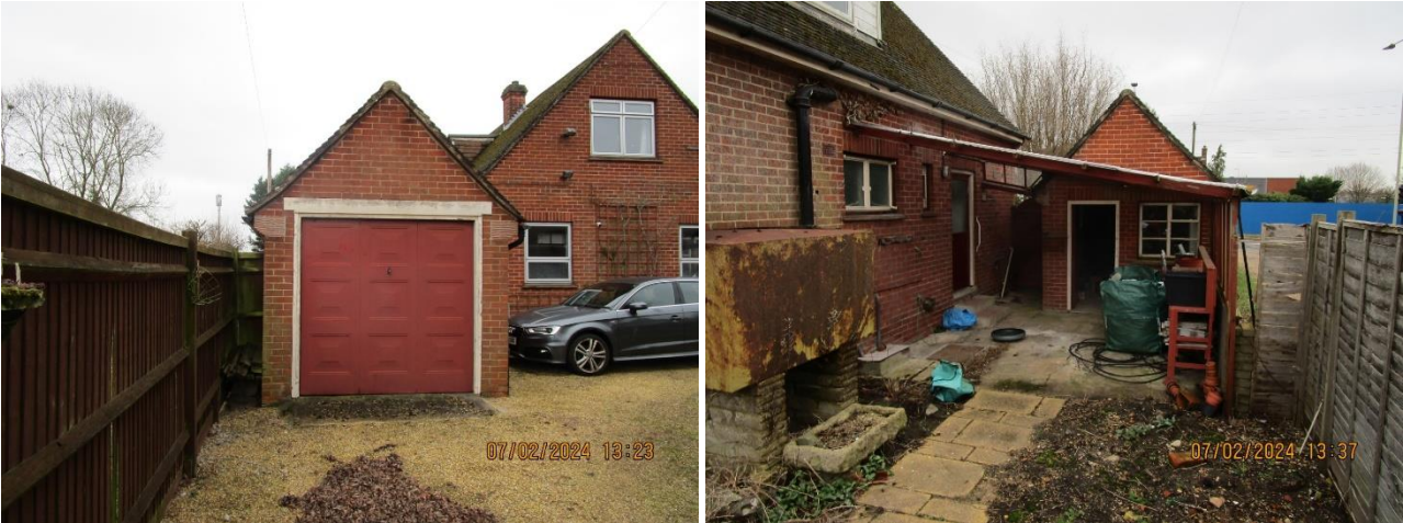
Photo 15 – Gap between the door frame and wall (garage), and Photo 16 – Gap between the wooden soffit and brick wall (garage)
