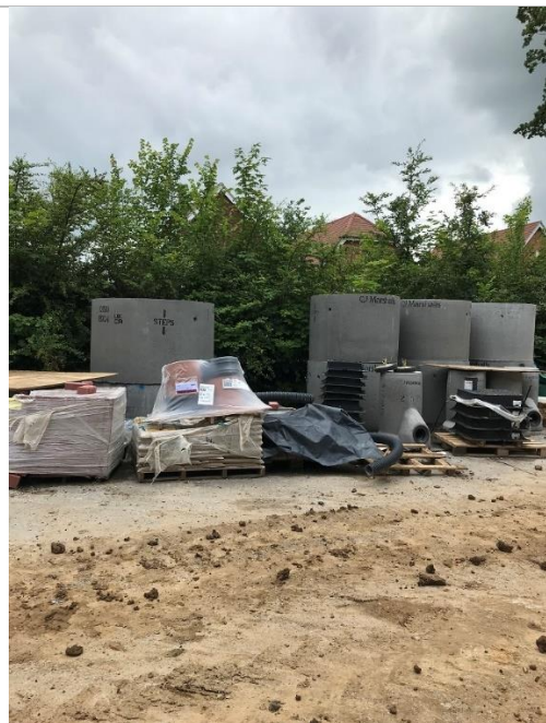
Photo 5. Car park used as storage area
