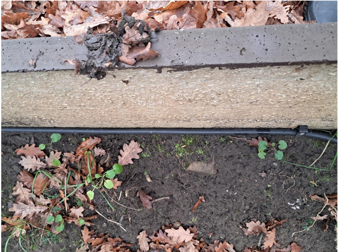
Figure 5 – Kickboard rests on pre-driveway construction ground levels – note the electric cable at base.
