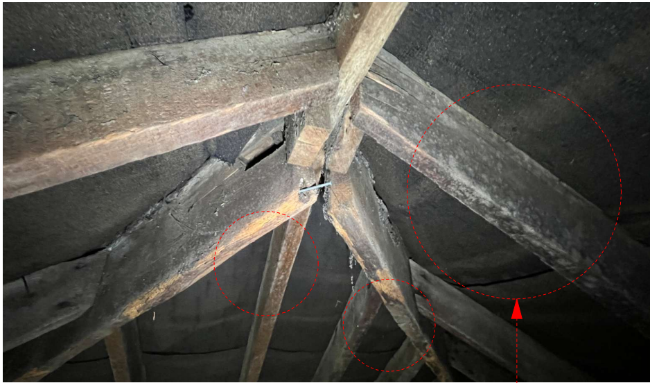
Mould growth present in almost every roof timber
