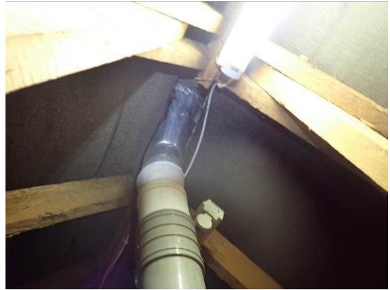
Photograph 17. Gap in felt around pipe at ridge.
