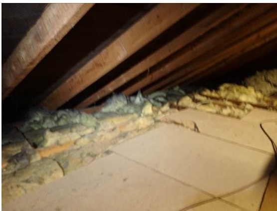
Photograph 18. Eaves partly blocked by fibreglass insulation.
