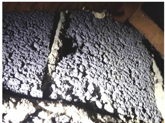
Photograph 19. Gaps around blockwork of front gable with old wasp nesting material.
