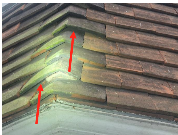
Photograph 12: Gaps beneath the hanging tiles on the northern elevation of B1.
