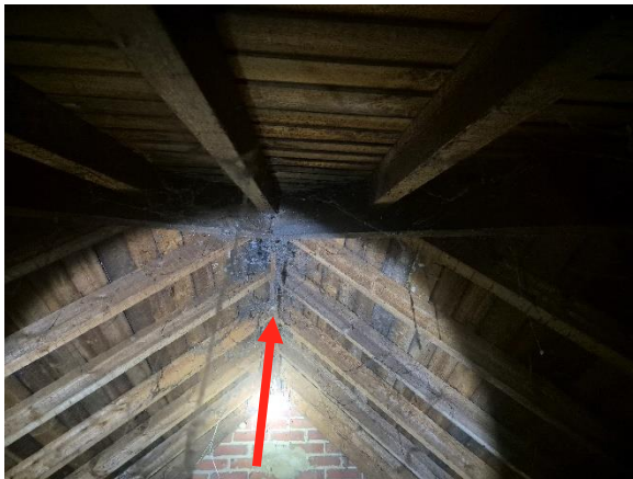
Photograph 9: Location of light ingress within the loft void of B1.
