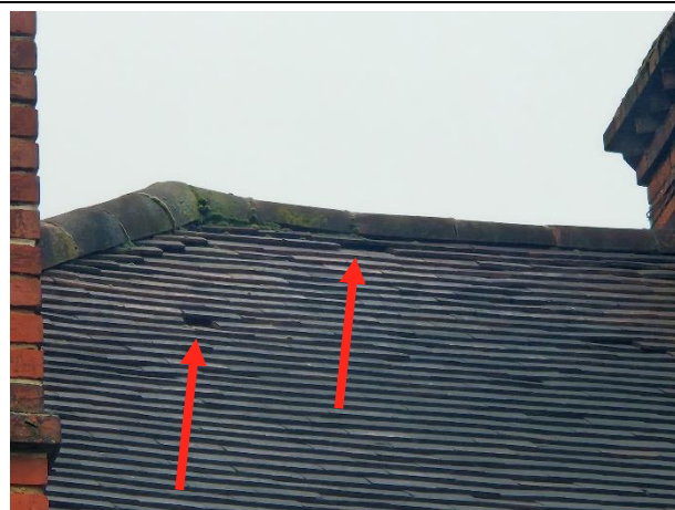
Photograph 13: Missing tiles on the southern elevation of B1.
