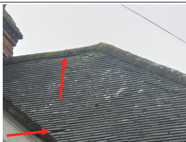
Photograph 11: Missing/ lifted tiles on the northern elevation of B1.
