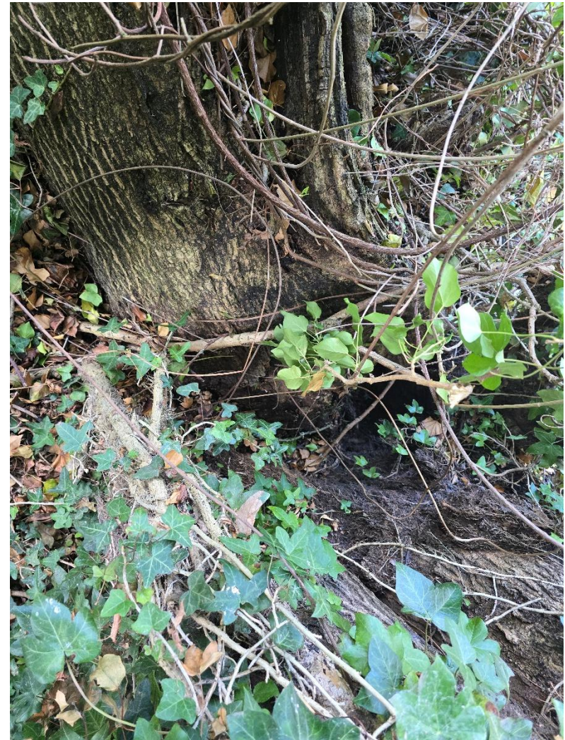
Photo 4 – Point of previous stem failure – trees within highway verge
