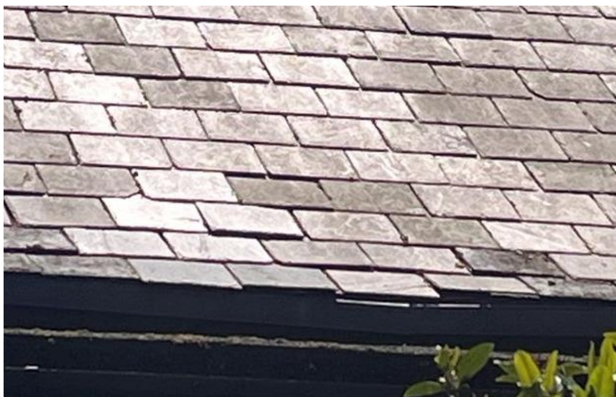
Plate 5: Image showing the gaps under the tiles on the northern elevation of B1 .
