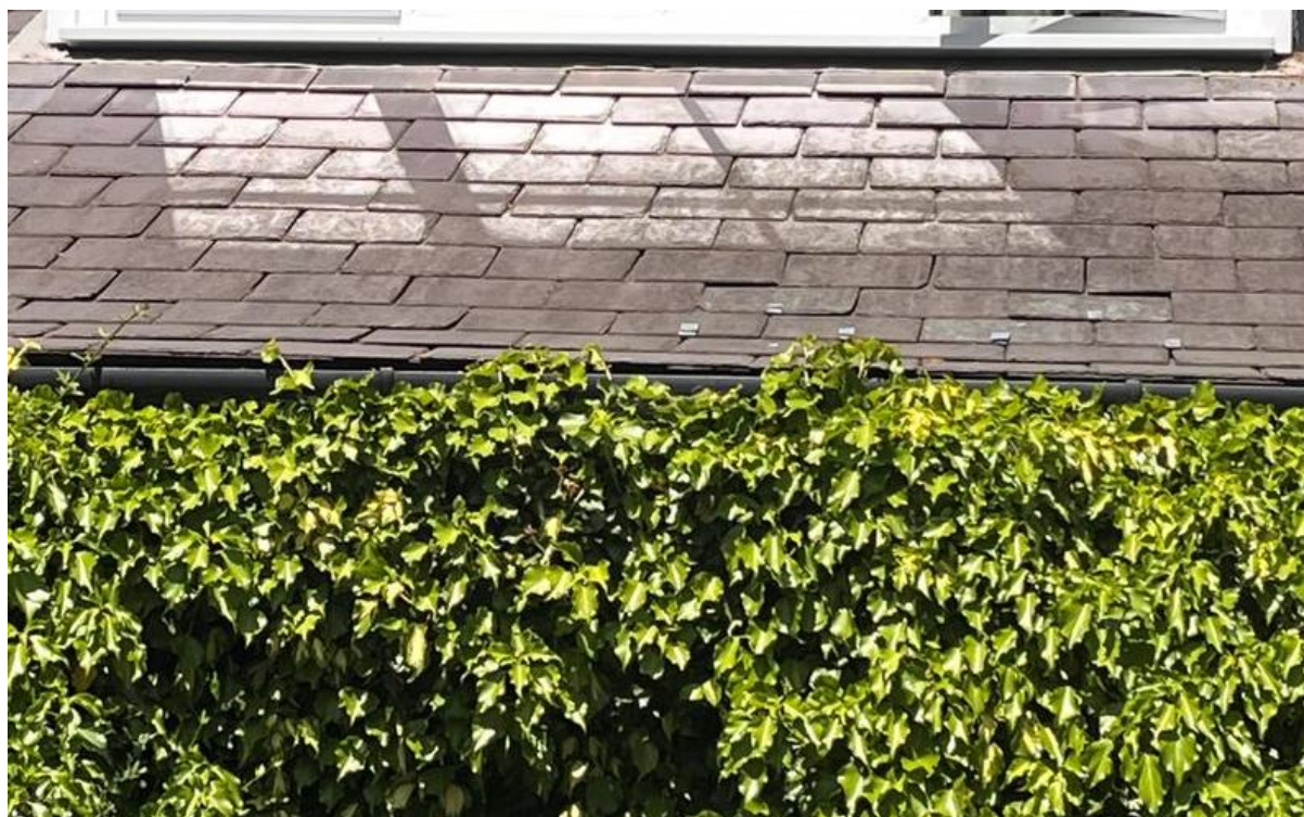
Plate 6: Image showing the gaps under the tiles on the southern elevation of B1 .
