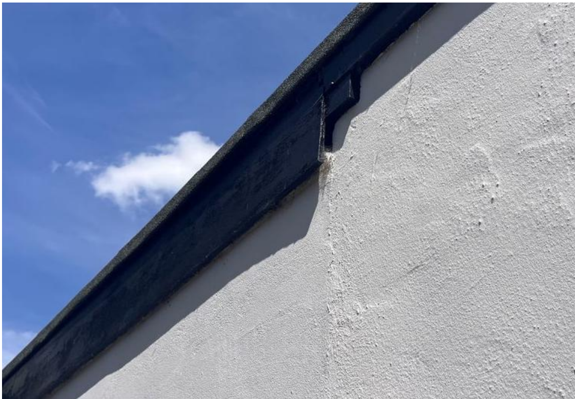
Plate 8: Image showing the gaps under the fascia on the western elevation of B1 .
