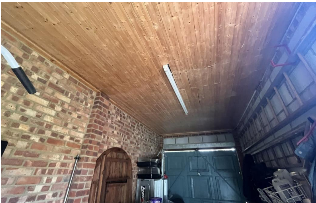
Plate 5: Image showing the gap above the garage door.
