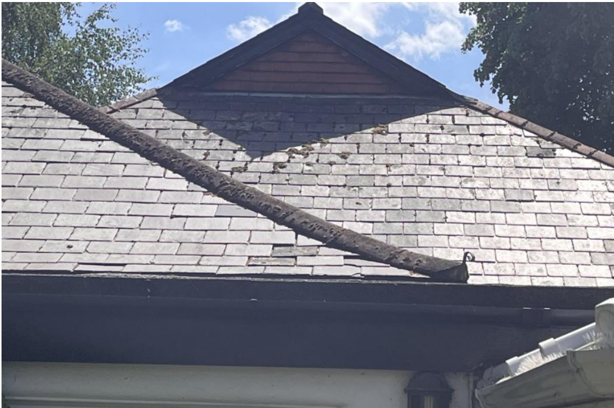
Plate 3: An image of the northern elevation of B1 , with the gaps under the roof tiles visible.
