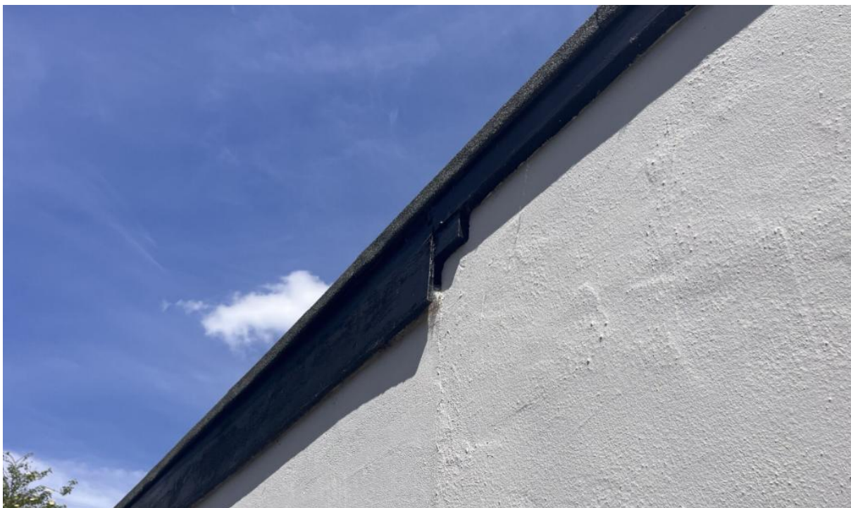
Plate 4: An image showing the gap behind the fascia on the western elevation.
