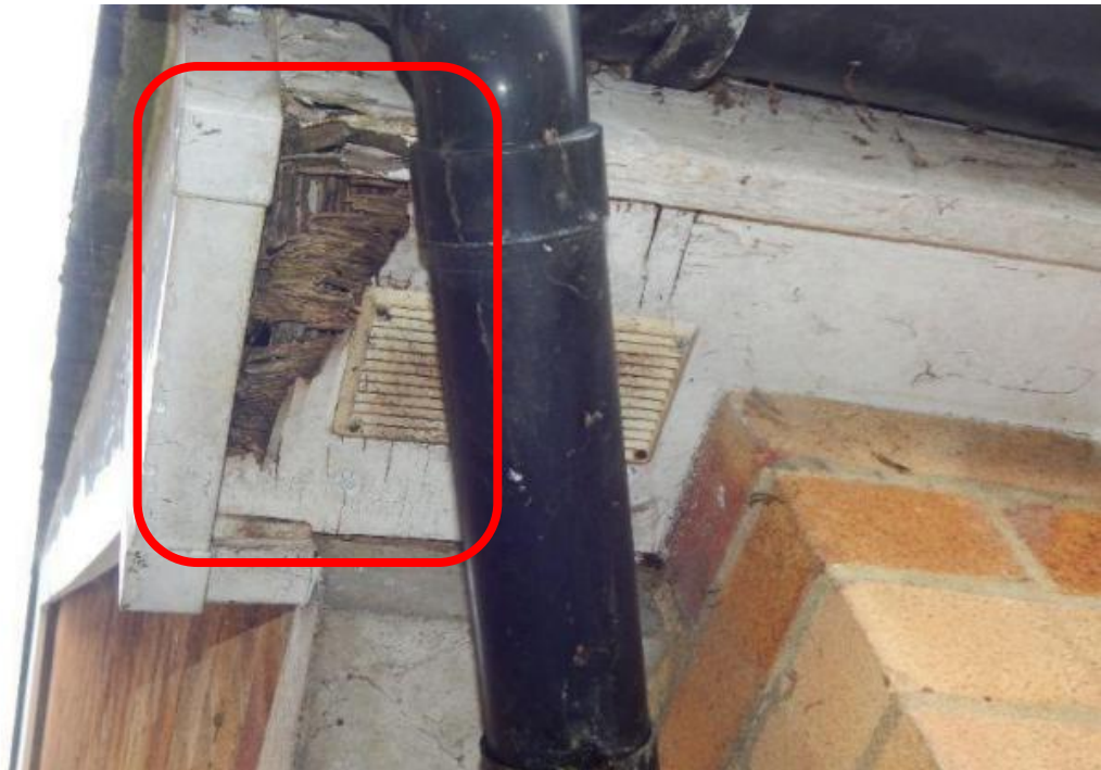
Image 7 – Damage to the eaves coverings which may provide further access opportunities for bats within
