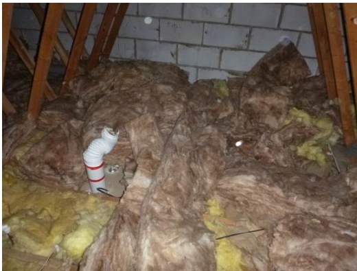
Photograph 9. Fibreglass insulation on floor.
