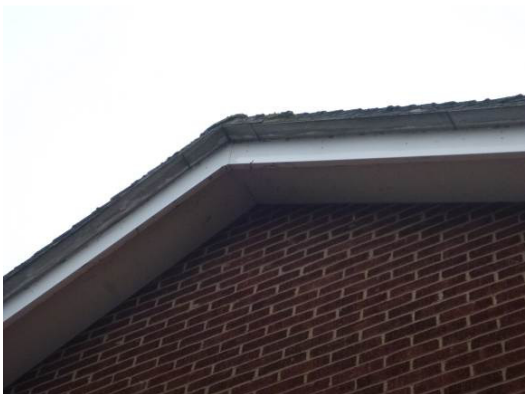
Photograph 6. Superficial crack in gable verge mortar (western elevation).
