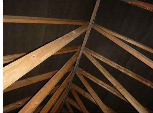
Photograph 8. Bitumen reinforced liner, lightly cobwebbed at the ridge.
