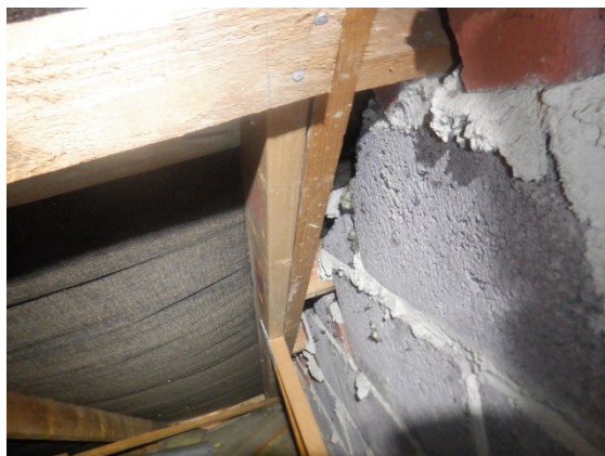
Photograph 15. Gaps along edge of the half-hipped gables.
