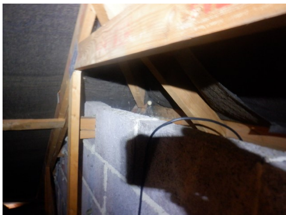
Photograph 14. Open gaps behind the half-hipped gables.
