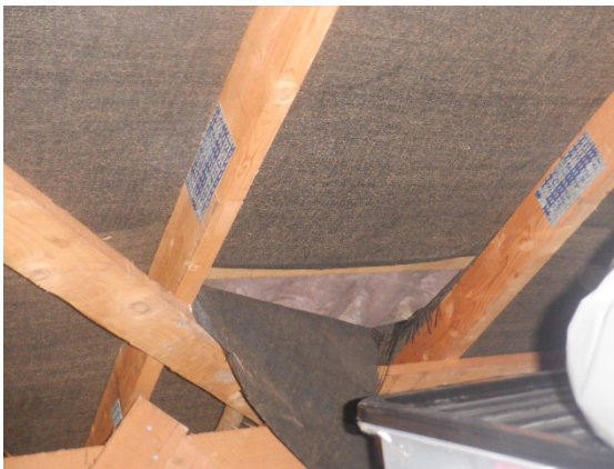
Photograph 12. Large tear in bitumen felt with underside of tiles visible.
