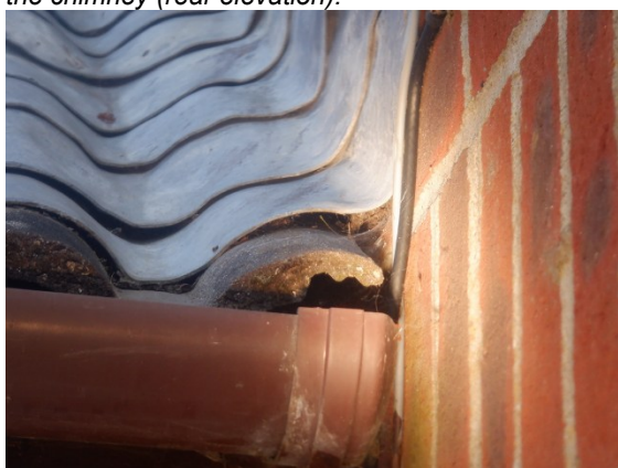
Photograph 8. Gap behind lead flashing filled with detritus (southwestern elevation).
