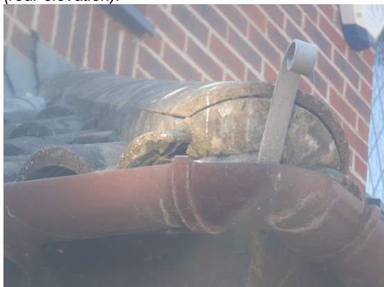
Photograph 5. Crumbling hip mortar with negligible suitability for roosting bats (front elevation).
