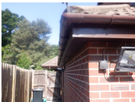
Photograph 10. Vented soffit sealed to brickwork along the existing extension (southwestern elevation).
