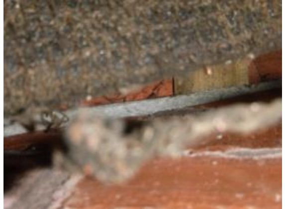
Photograph 20. Tear in bitumen felt at northwest corner (Garage void).
