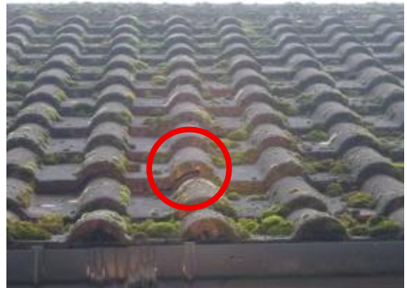
Photograph 4. Slightly lifted tile; gaps of limited extent (front elevation).
