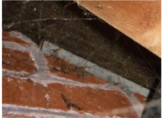
Photograph 22. Gaps along the edges of the brickwork gable (Garage void).
