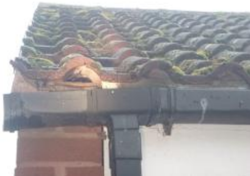
Photograph 3. Damaged tile partially blocked by guttering (front elevation).
