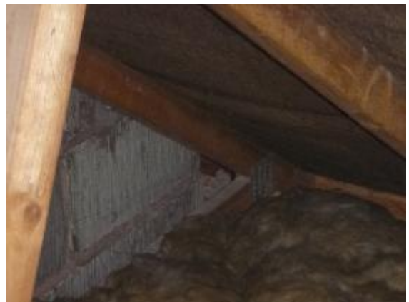
Photograph 18. Gaps at the corner of the north blockwork internal wall (Roof void 1).
