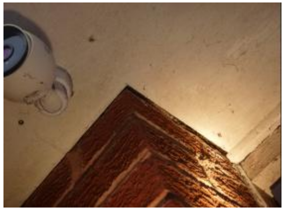
Photograph 13. Painted timber soffit tight to the single-storey extension (front elevation).
