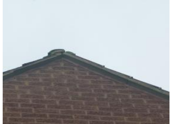
Photograph 8. Crumbling verge mortar at the apex of the eastern gable (eastern elevation).
