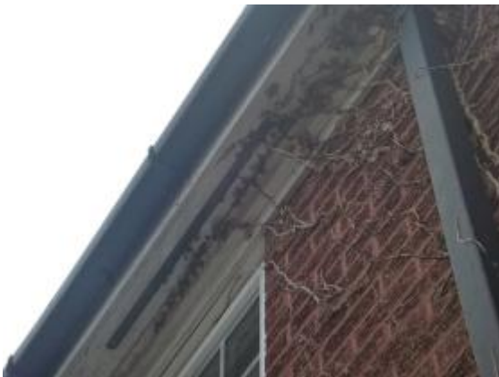
Photograph 12. Painted timber soffit sealed to the property (rear elevation).
