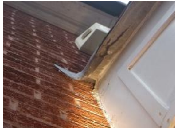
Photograph 10. Gap behind lead flashing above bay window (north elevation).
