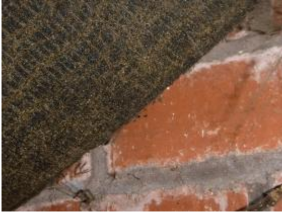
Photograph 19. Loose bitumen felt along the north brickwork gable (Garage void).
