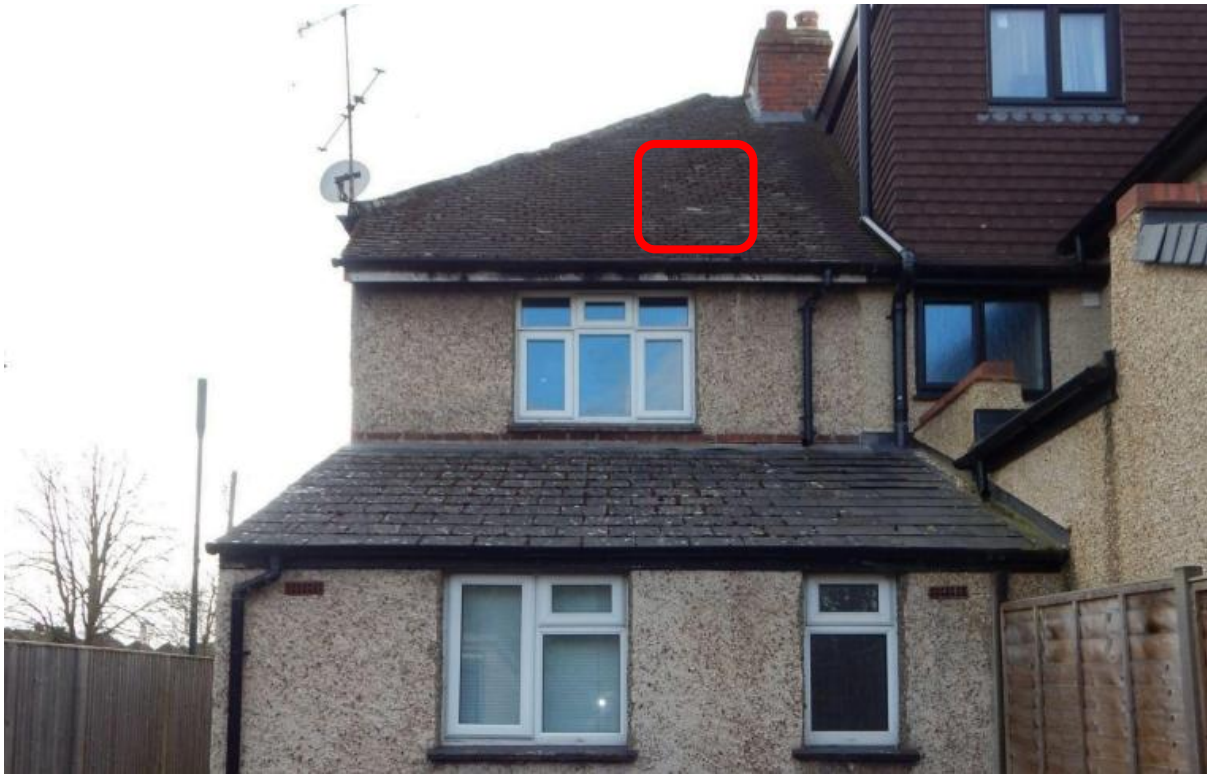
Image 3 – West facing elevation n of the property where gaps of adequate proportions to offer likely shelter/access opportunities for bats were observed within the tiled coverings
