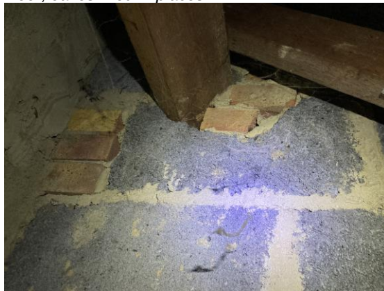
Photograph 12. Gaps around support timber, no daylight visible.
