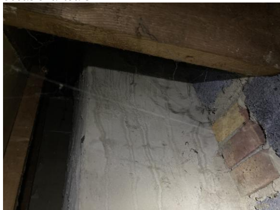
Photograph 11. Chimney tight and heavily cobwebbed.
