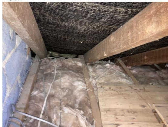
Photograph 10. Fibreglass insulation on part-boarded
