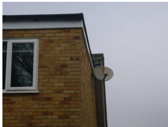
Photograph 6. Flat roof fascias tight to the brickwork.
