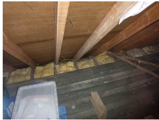
Photograph 15. Roof void open at the eaves.
