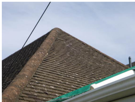
Photograph 5. Occasional missing hip mortar (southeast elevation).
