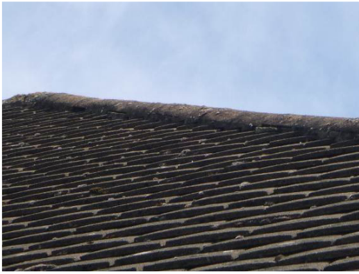
Photograph 6. Occasional missing hip mortar (front elevation).
