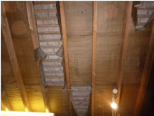
Photograph 16. Large tears in the roof lining.
