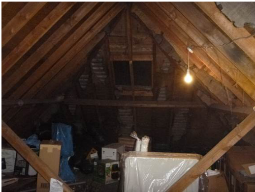
Photograph 13. Large roof void.
