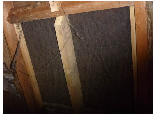
Photograph 21. Old chimney removed and tight bitumen felting.
