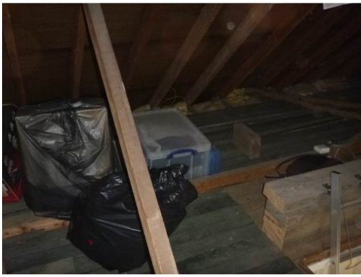
Photograph 20. Mostly boarded floor.
