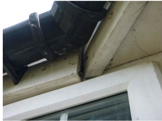
Photograph 9. Superficial gap in fascias on bay window (front elevation).
