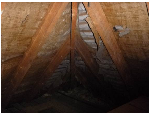
Photograph 18. Large tears in the roof lining at the hip of the roof.
