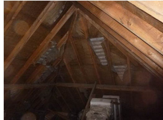
Photograph 17. Large tears in the roof lining at the hipped ends.
