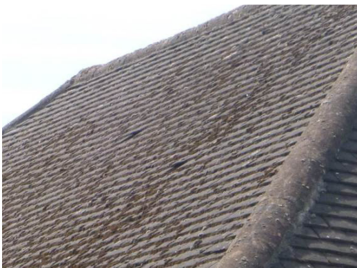
Photograph 4. Two missing roof tiles (northeast elevation).
