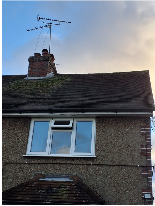
Photograph 2. Uneven clay roof tiles (front elevation).
