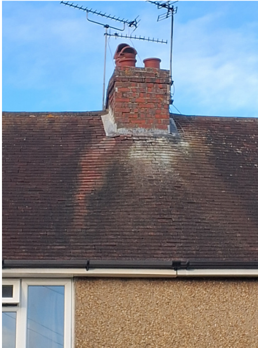
Photograph 1. Uneven clay roof tiles at the base of the chimney (rear elevation).
