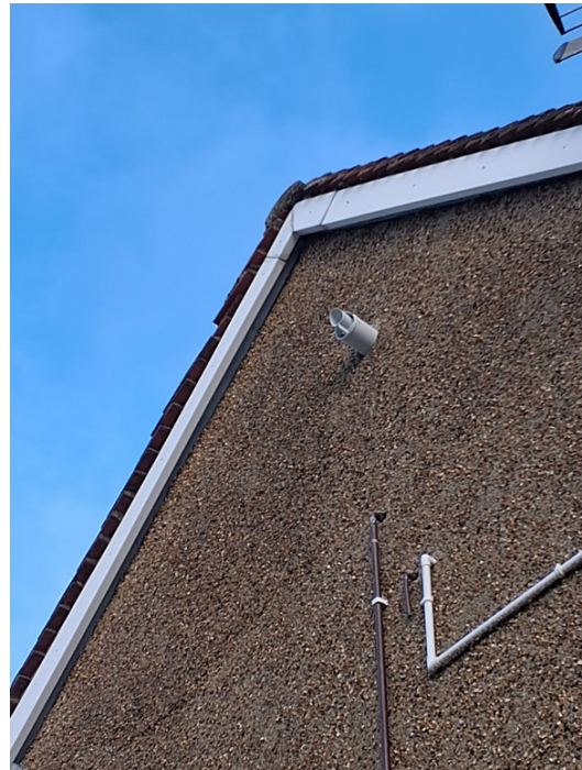
Photograph 7. Gap between gable and uPVC fascia (west elevation).
