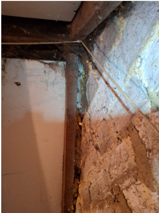
Photograph 14. Heavily cobwebbed gap at the apex of the gable.
