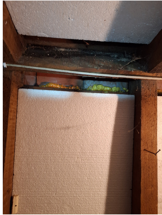
Photograph 11. Unlined ridge with expanding foam visible.
