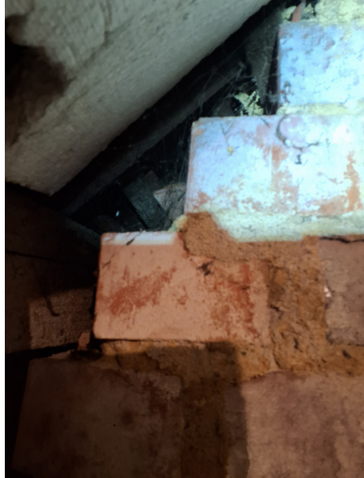
Photograph 13. Open gap within brickwork party wall, allowing access to neighbouring void.
