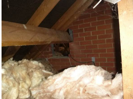
Photograph 15. Hole into side extension (roof void).
