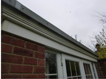
Photograph 9. Tight fascias on rear extension (rear elevation).
