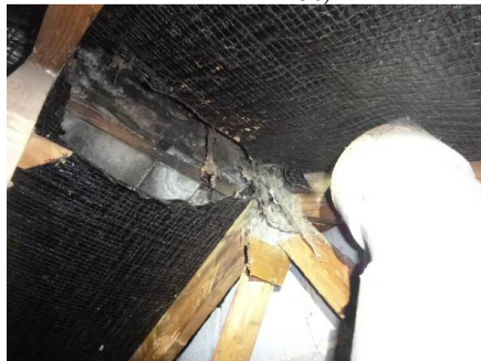
Photograph 13. Tear in roof lining at ridge (roof void).
