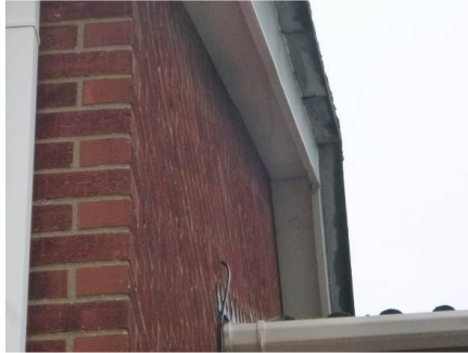
Photograph 6. Potential bat access behind gable soffits (north-eastern elevation).
