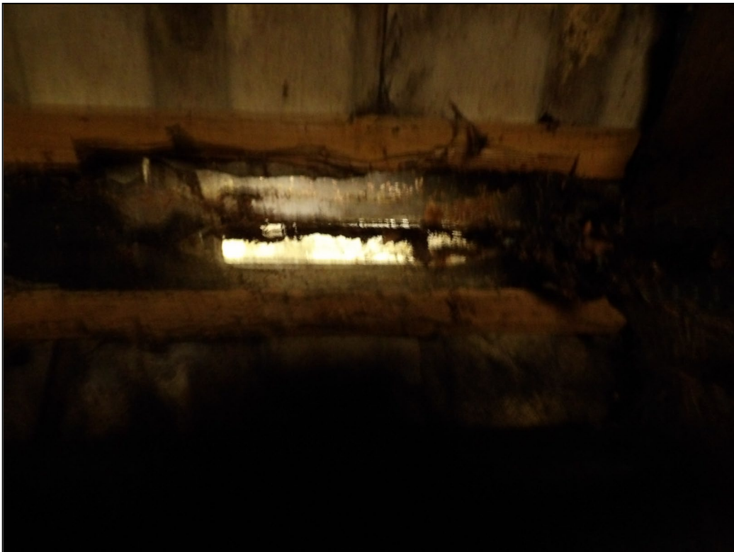
Figure 13. Light ingress through open roof vent. 216b Nine Mile Ride, Wokingham. 21.01.25
