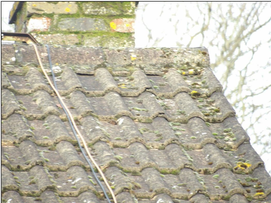
Figure 4. Example raised roof tiles. 216b Nine Mile Ride, Wokingham. 21.01.25
