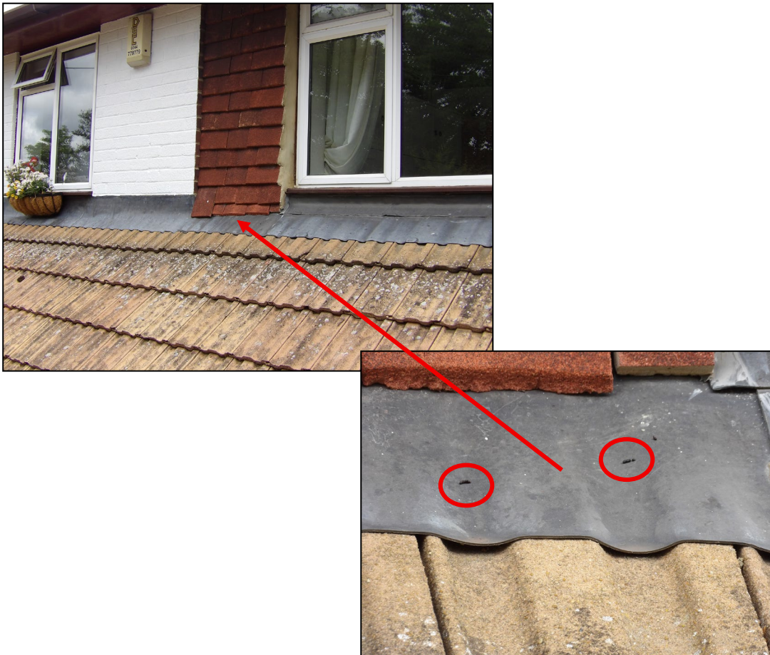
Figure 12. Bat droppings on front elevation. 104 Reading Road, Finchampstead. 10.06.25
