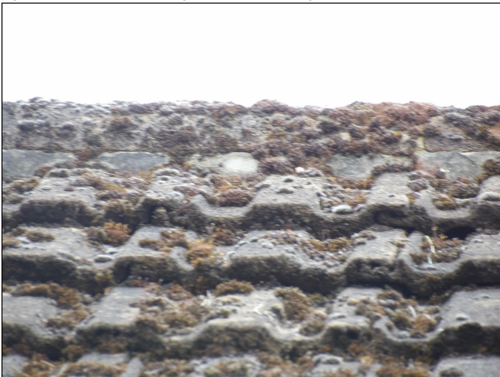
Figure 6. Example sealed ridge tiles. 104 Reading Road, Finchampstead. 10.06.25
