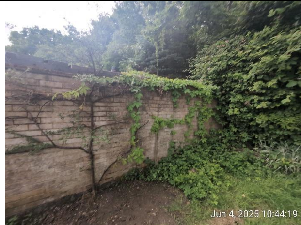
Figure 13: site northern wall with virginia creeper
