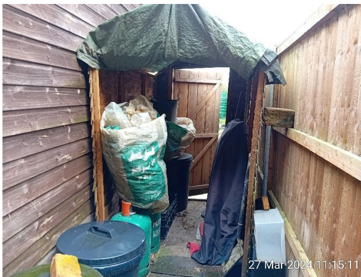
Figure 10: B6, with back panel removed
