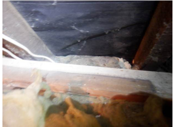
Photograph 15. Eaves partially filled.
