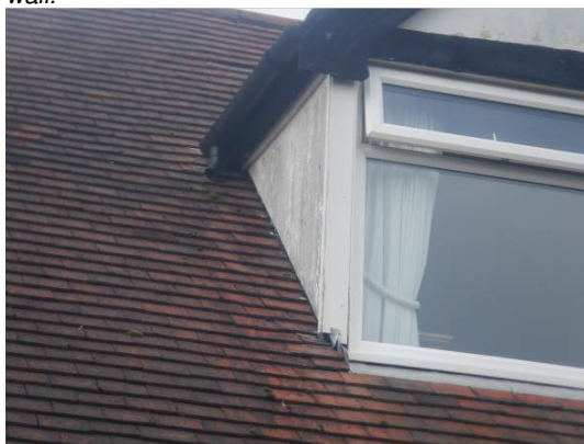
Photograph 9. Plastered walls tight on the rear dormer window.
