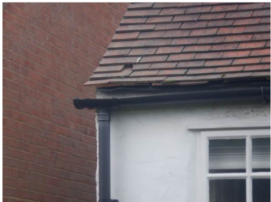
Photograph 3. Cobwebbed gap under roof tile on the rear elevation.
