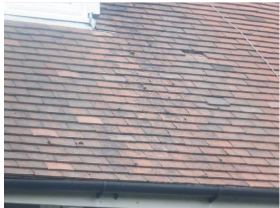
Photograph 4. Gap of limited extent under the roof tile on the rear elevation.
