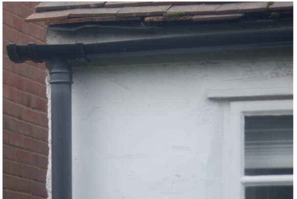
Photograph 8. Soffits obscured by guttering on the rear elevation.
