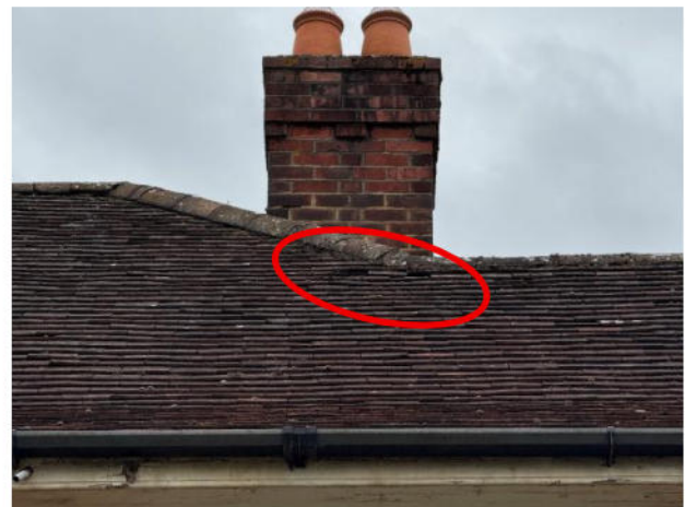
Gaps under roof tiles on northern aspect.
