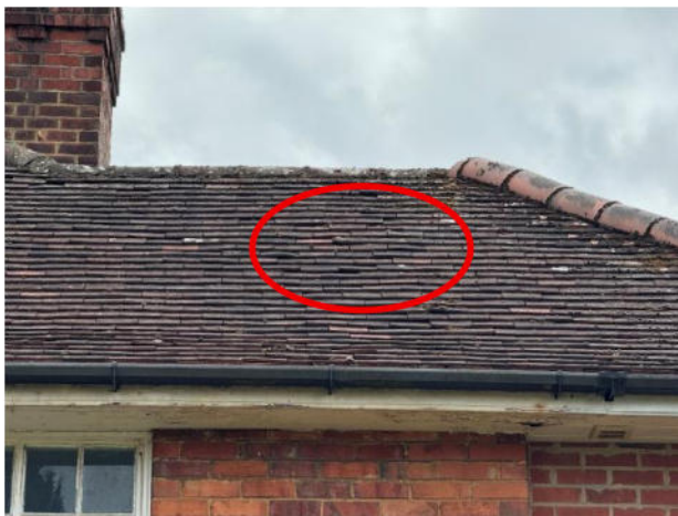
Gaps under roof tiles on northern aspect.
