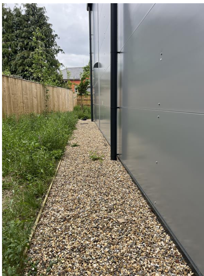
Figure 4.3: Site photo showing screening loss
