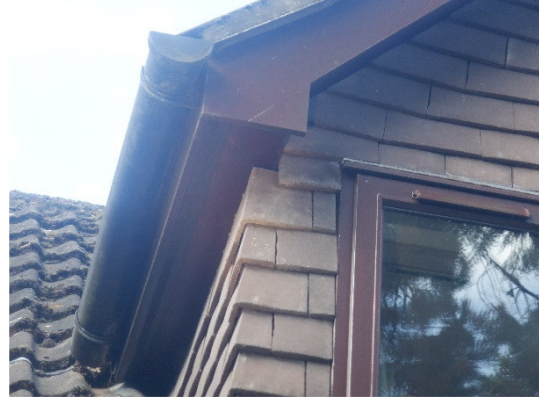
Photograph 10. Gaps in the tiles around the top edges of the window frames (eastern elevation).
