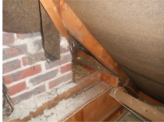
Photograph 20. Bird nesting material at the eaves in the roof void.
