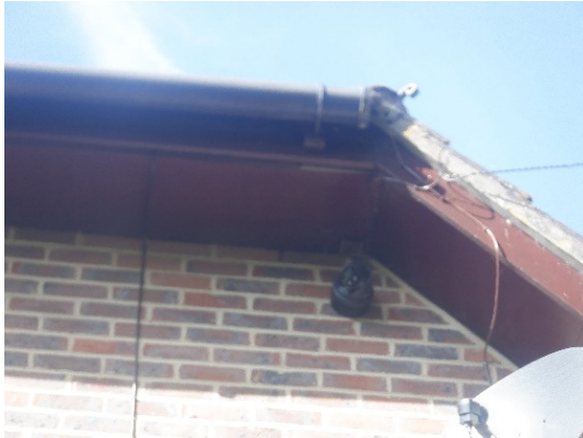
Photograph 5. Gaps behind soffit boxes at hipped ends (eastern elevation).
