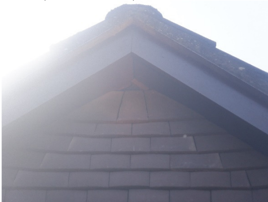
Photograph 11. Missing tile at apex of front eastern-most dormer window (front elevation).
