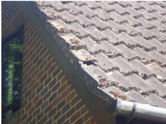
Photograph 3. Broken tile (rear elevation).
