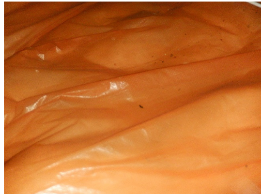
Photograph 22. Medium-sized bat droppings within the void.
