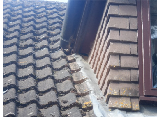
Photograph 12. One of the large gaps present in the roof junction of a dormer window (eastern elevation).
