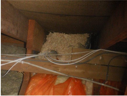
Photograph 19. Wasp nest present in the eastern end of the roof space.
