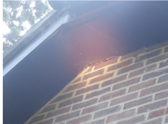
Photograph 6. Large, cobwebbed gap at hipped end (northern elevation).
