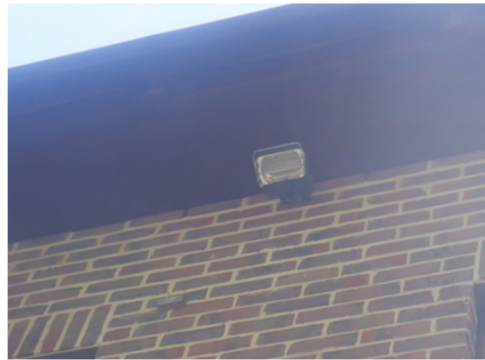
Photograph 8. Slits in a few bricks on the western elevation.
