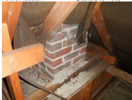
Photograph 18. Heavily cobwebbed chimney (roof void).
