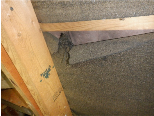
Photograph 14. Loose bitumen felt (roof void).
