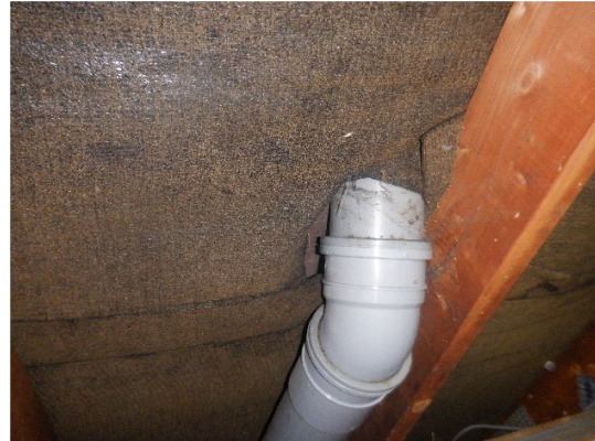
Photograph 15. Loose bitumen felt around the chimney at the internal brickwork wall (roof void).
