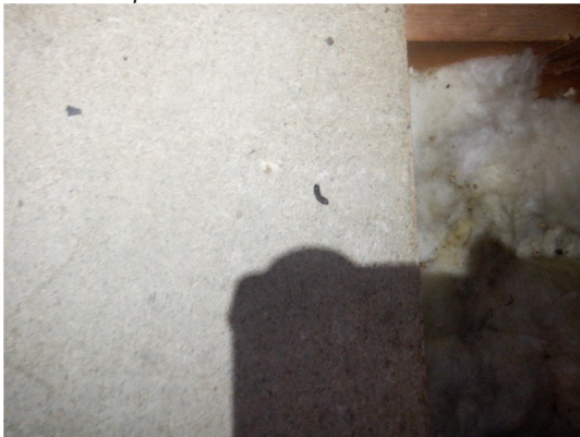
Photograph 21. Medium-sized bat droppings within the void.
