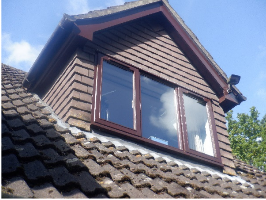
Photograph 9. Lifted corner hanging tiles on dormer window (eastern elevation).
