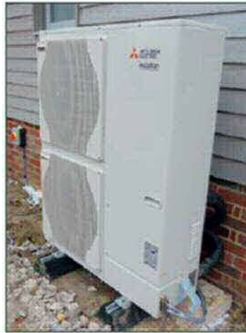
Photograph 1 - Typical Air Source Heat Pump
