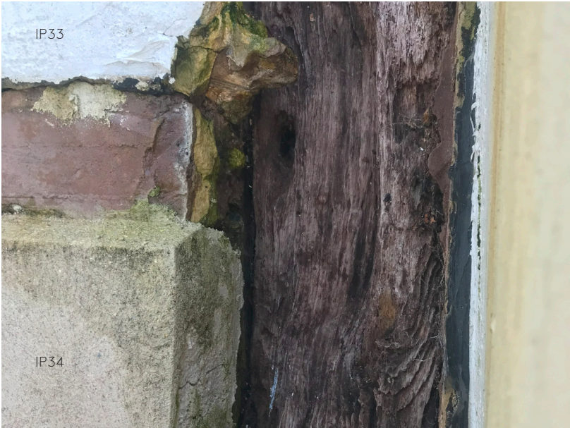
07 DECAY OF TIMBER POST (LEFT OF CH02)) NTS
