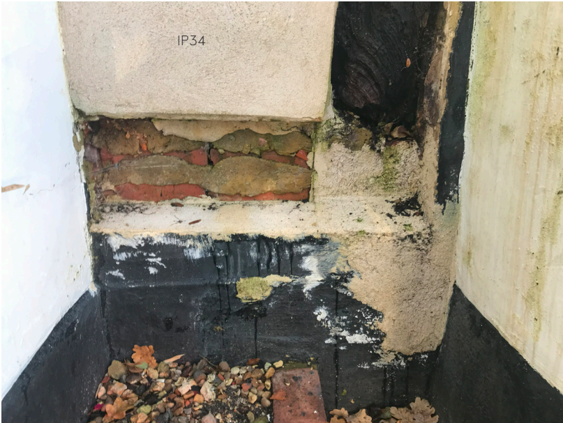
06 BRICK REVEALED BEHIND MISSING BOARDING NTS
