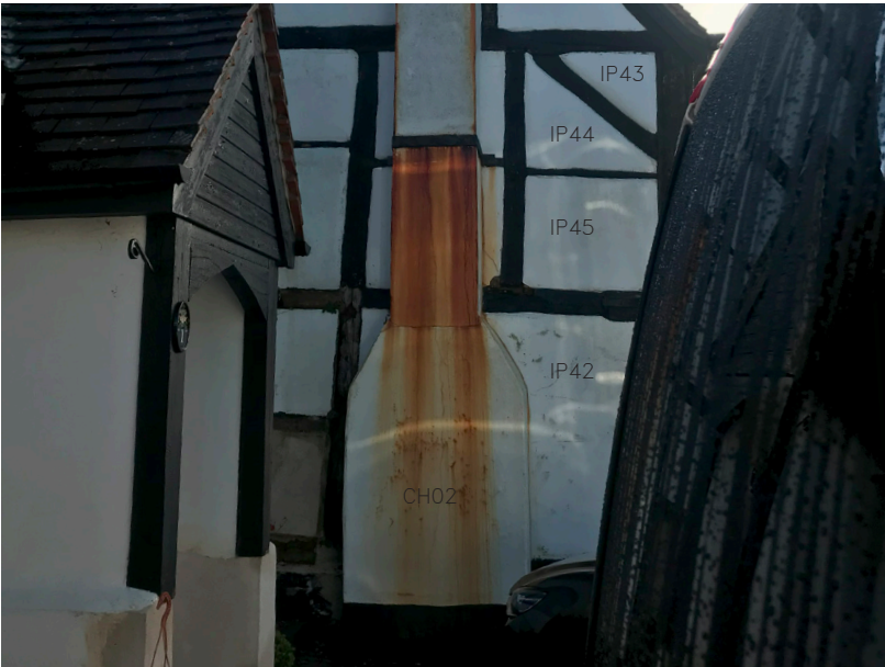
08 RUST STAINING TO PAINTED FINISH ON CH02 NTS
