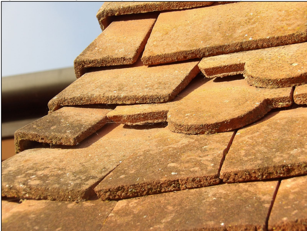
Figure 8. Example gaps in hanging tiles. 98 Broad Hinton, Twyford. 03.12.24
