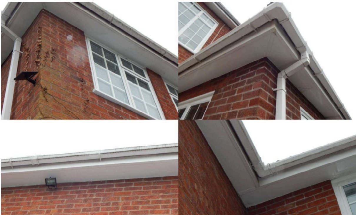
Image 6 – Close views of the eaves covering to show examples of condition
