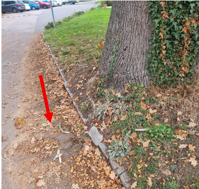
Photograph 7. Damage to edging stones and cracking/lifting of tarmac.
