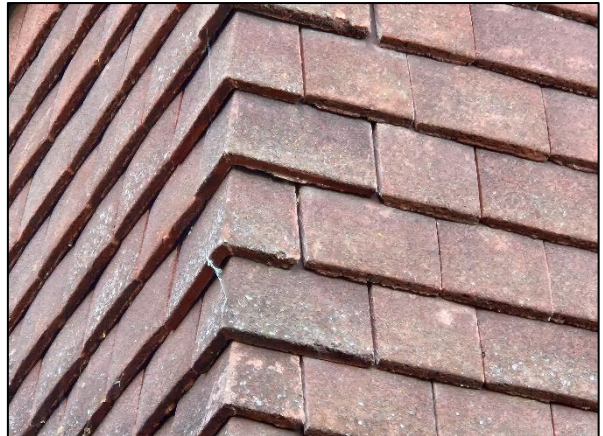
Photo 8: Tight hanging tiles on dormer.
