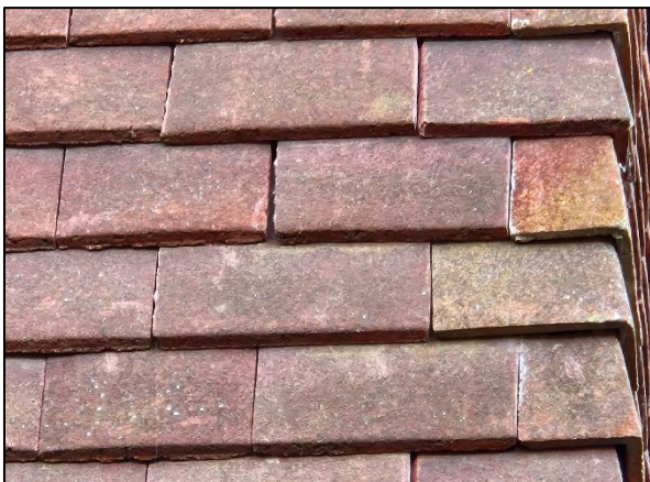
Photo 9: Tight hanging tiles on dormer.
