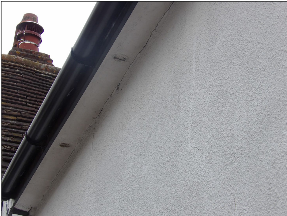
Figure 10. Example sealed soffits and fascias. 98 Pitts Lane, Earley. 24.06.25
