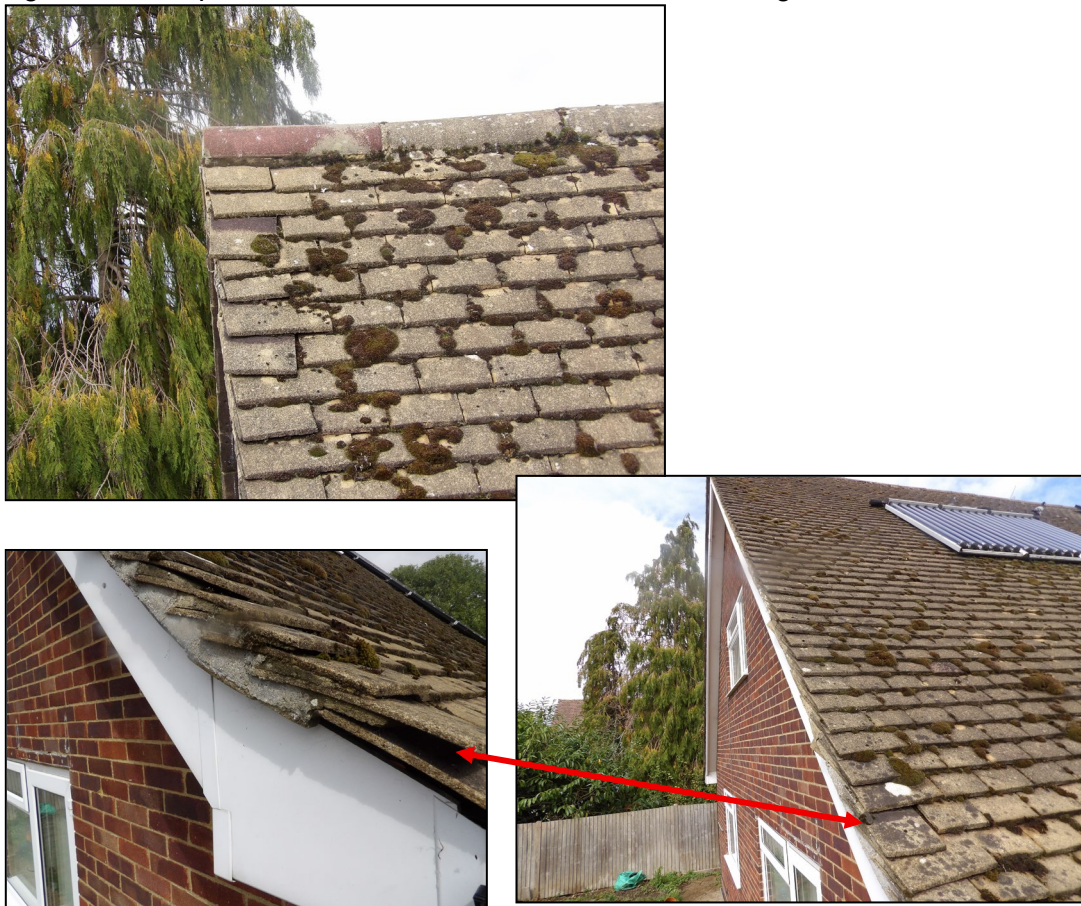
Figure 4. Examples moved roof tiles. 3 Garde Road, Sonning. 02.09.25
