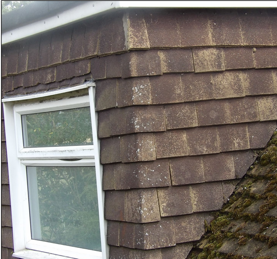
Figure 10. Example moved hanging tiles on dormer. 3 Garde Road, Sonning. 02.09.25
