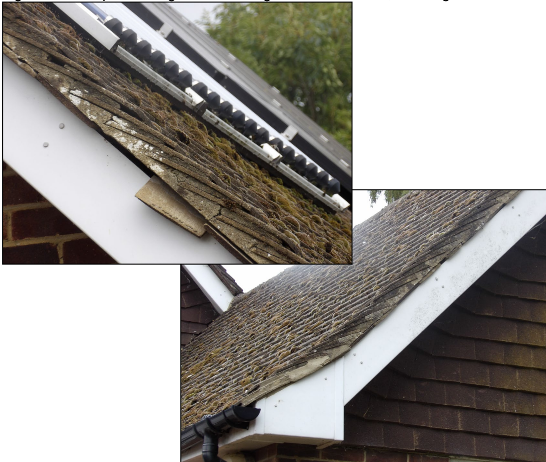
Figure 6. Example missing mortar in verges. 3 Garde Road, Sonning. 02.09.25
