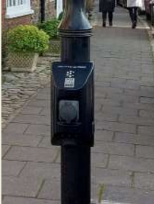
FIGURE 215 STANDARD LIGHTING COLUMN WITH EV CHARGING POINT
