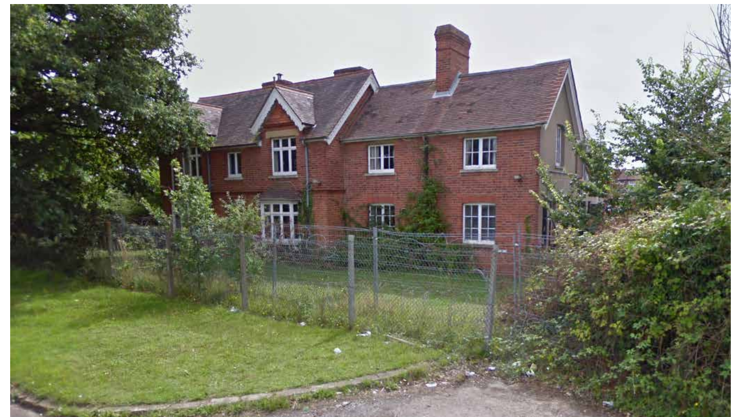
Figure 2.14 Image from 2009 showing the concrete render which has resulted in sustained damp within the building
