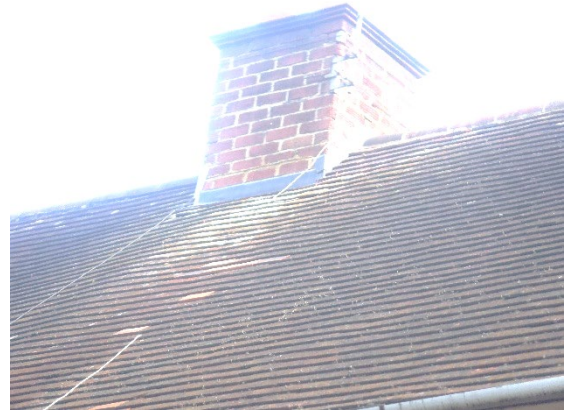
Photograph 4. Uneven roof tiles around chimney.
