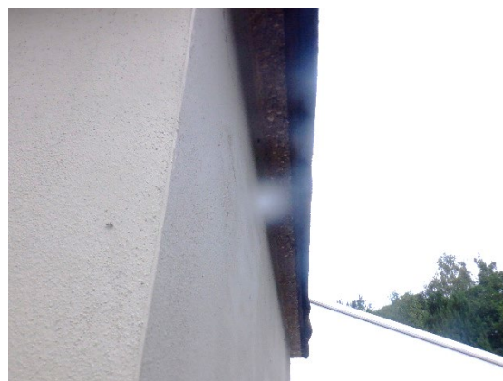
Photograph 6. Superficial gap beneath bitumen felt of single storey side extension.
