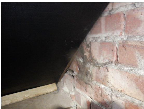
Photograph 11. Gap in brickwork at south eastern gable end.
