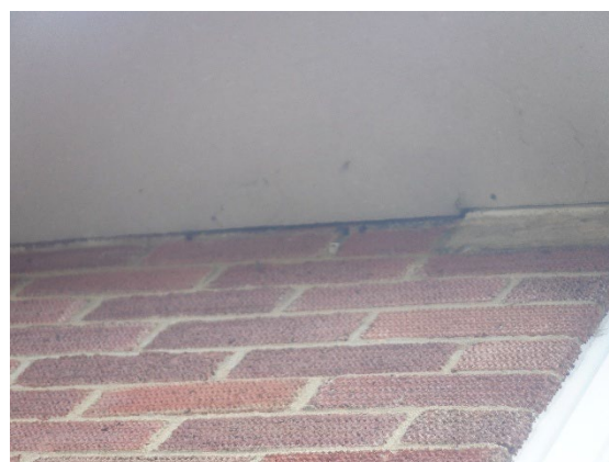
Photograph 8. Gap behind board soffits (front elevation).
