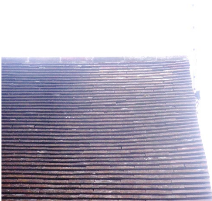
Photograph 3. Gaps beneath verge tiles (front elevation); tightly fitted ridges.
