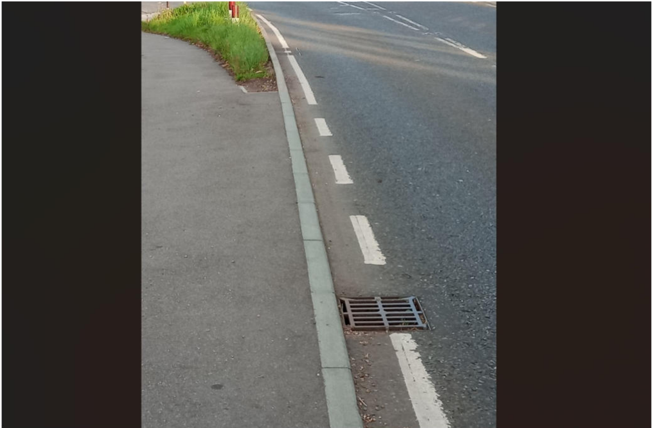
Image 10 - the (insufficient) three highway gulley-openings serving Bridge Cottages:
