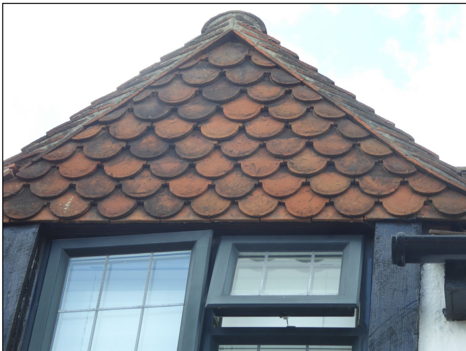
Figure 7. Hanging tiles on front elevation. 75 Pitts Lane, Earley. 05.06.24
