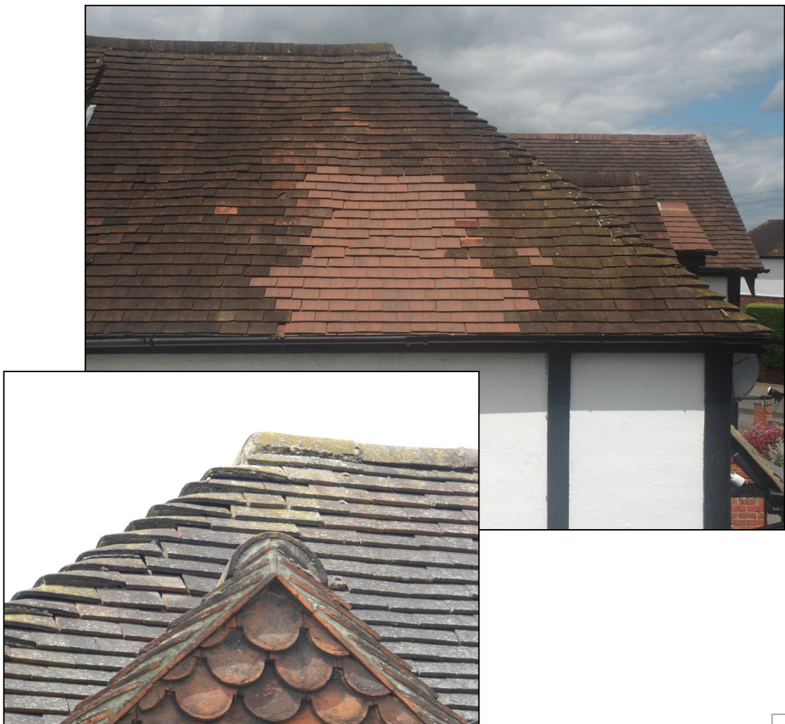
Figure 5. Lifted hip and roof tiles on east and south elevation. 75 Pitts Lane, Earley. 05.06.24
