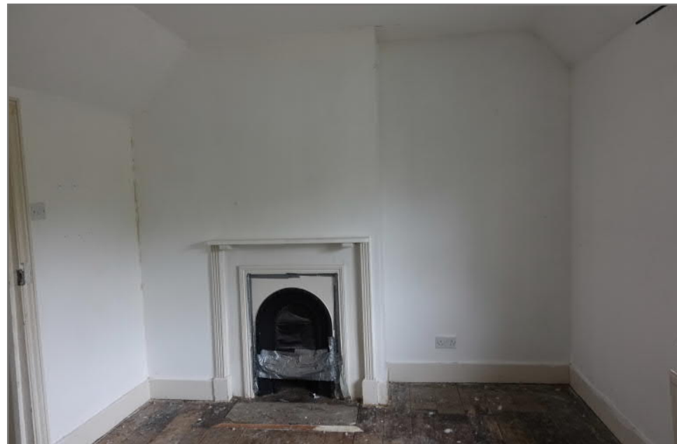
Image 61: View north of C19 gable extension (northeast room) - fireplace missing
