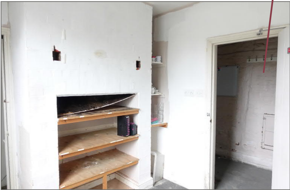
Image 40: Redundant chimney breast - no through roof chimney
